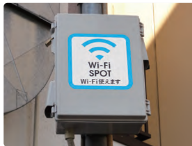
Wi-Fi Access Point
